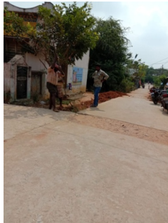
Figure 5.8: Condition of Roads
