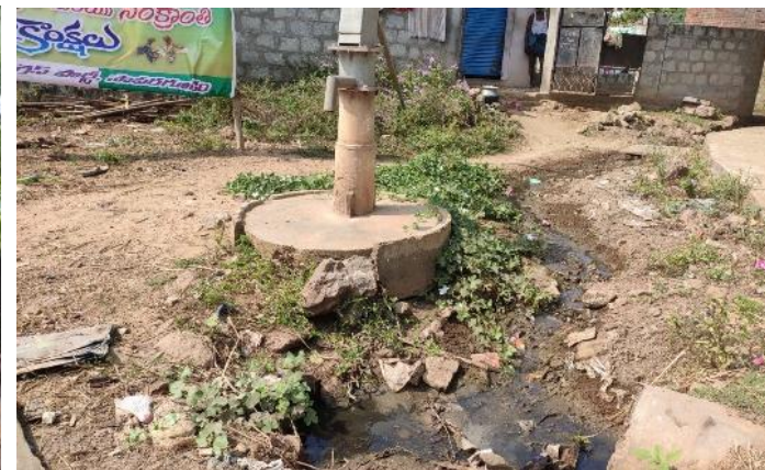
Figure 4.6: Hand Pump Condition
