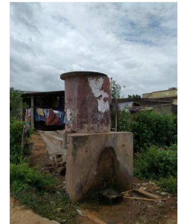
Figure 5.11: Condition of Water supply
